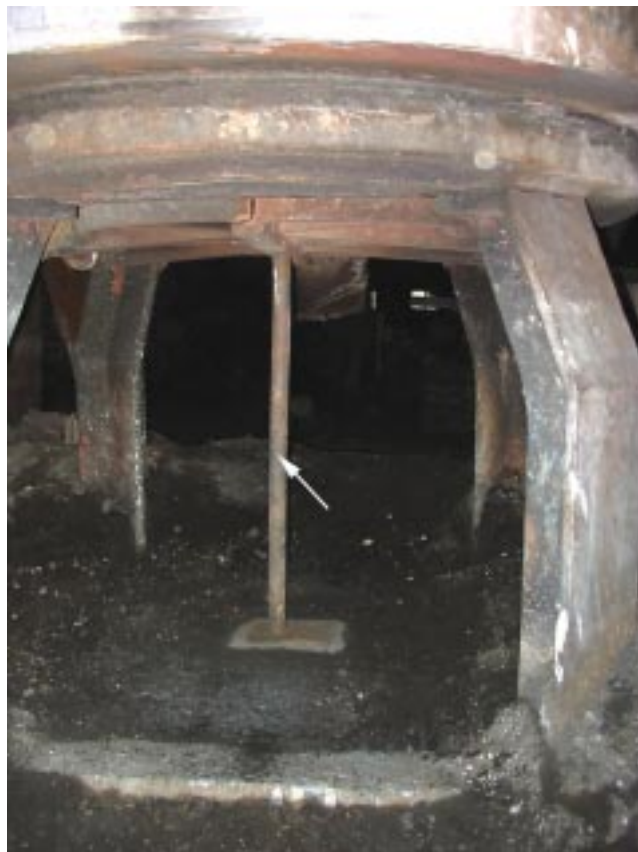
Photo 10. Bottom doors of cupola propped shut with a length of iron pipe (see white arrow).
