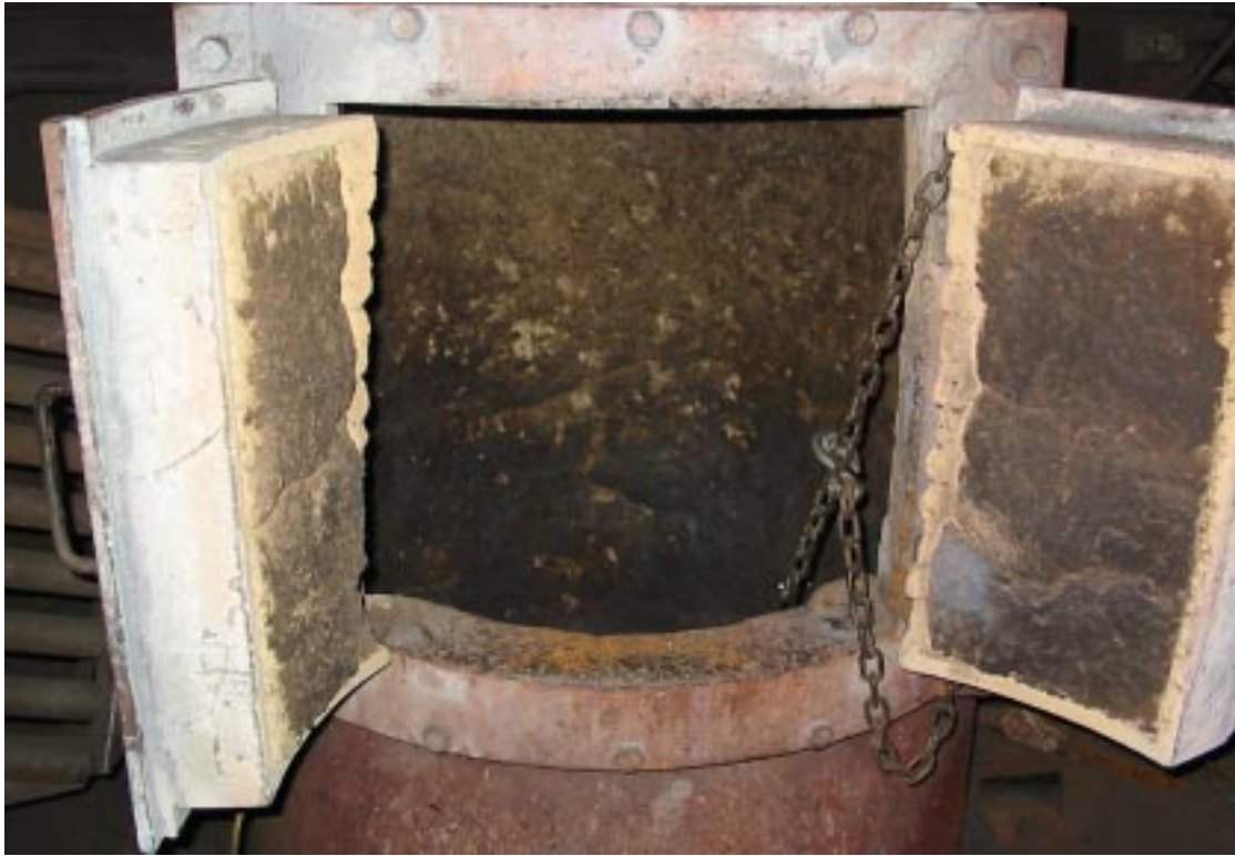
Photo 7. The charging doors on the cupola.
