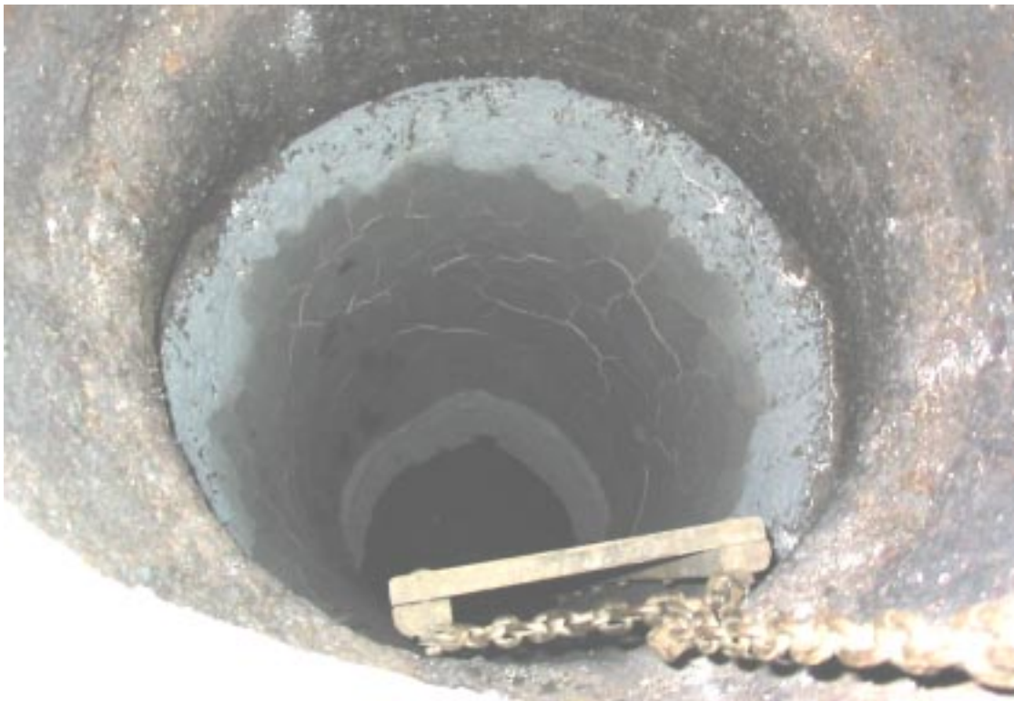
Photo 8. Looking down into the cupola through the charging doors. Notice the layer of daub. (The chain is supporting a wooden ladder used to enter the cupola to level sand on the bottom doors.)
