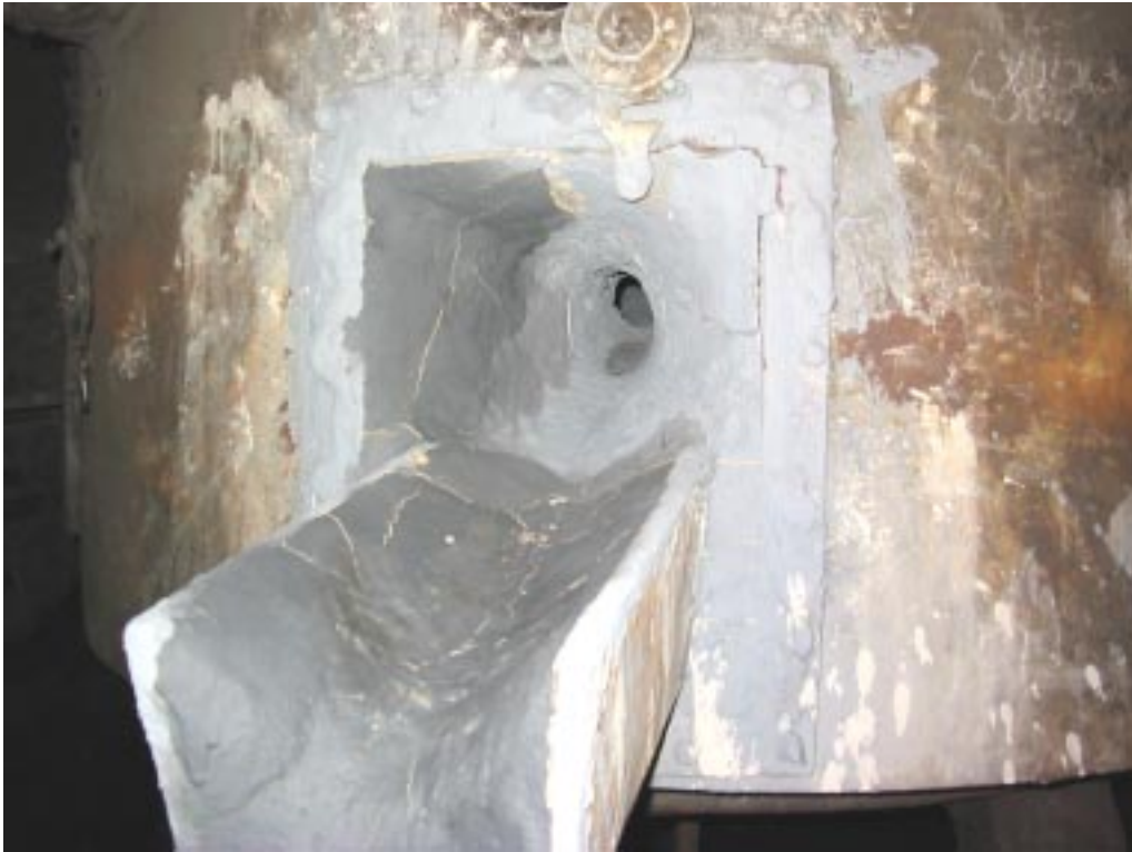
Photo 9. Slag hole and spout of the cupola. Note the fresh coating of daub.
